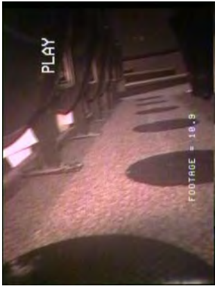
Figure #9 Gallery piping exhaust close-ups
