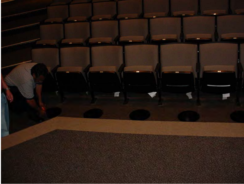
Figure #3 Gallery exhaust vents within the theatre
