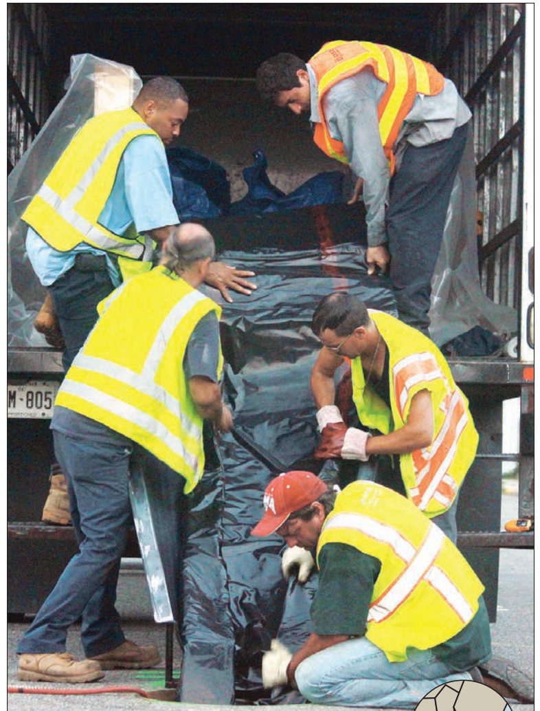
The Lanzo Lining Services and Advance Underground Inspections crews pull a 24-inch liner with project superintendent Steve Carbeck (red hat), who was on hand 24/7 with all operations. (Photos courtesy of Pacific Multilining)
