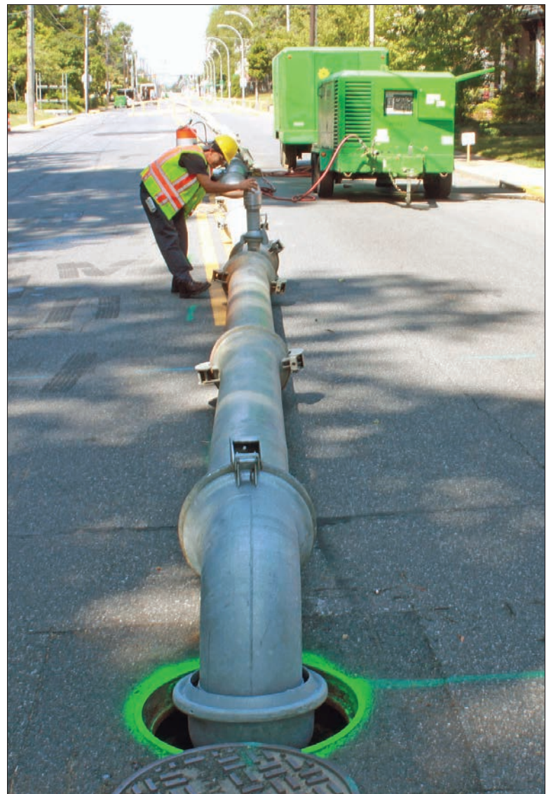
At the end of the mile-long bypass system, a crew member checks the pressure and releases a small amount of air so that the bypass system flows with ease.
