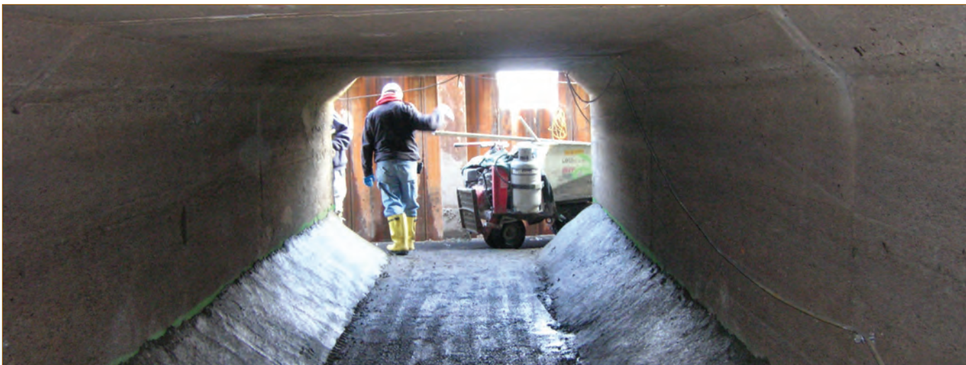
The Joe Campau B 10 Outfall installation that rehabilitated 3,600 lf of a rectangular box culvert in Detroit pushed the boundaries of pipe rehabilitation.
