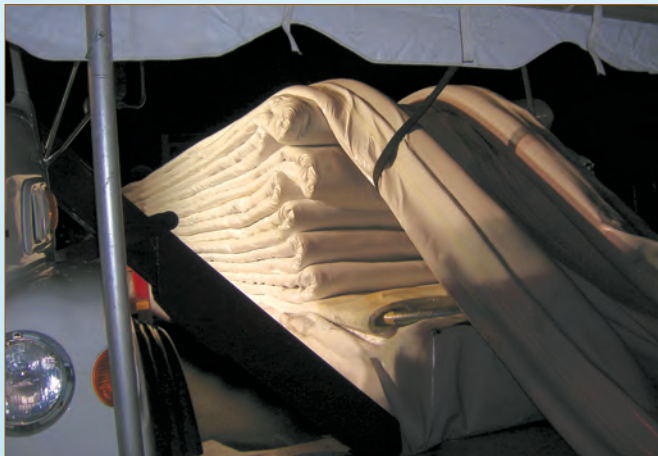
The over the hole inversion technique is used when the tub and resin weigh too much to factory impregnate and haul to the site. Instead, a makeshift plant is assembled over the pit, or hole.
